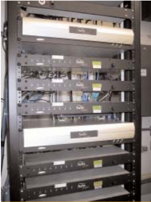
Rack of AudiaFLEX units and AudiaEXPI's used in the installation.
