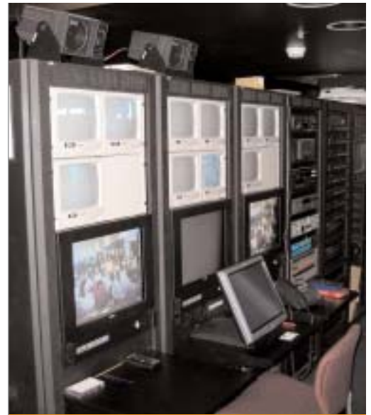
Hansen Hall's control room.
